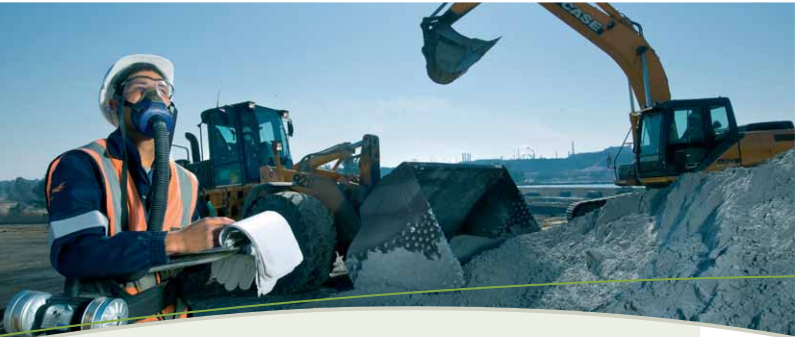
Keeping records of loads of ash to track and control blending ratios at the tarpit blending project at Sasolburg, where fine and coarse ash are blended with tar to stabilise the tarpits.
