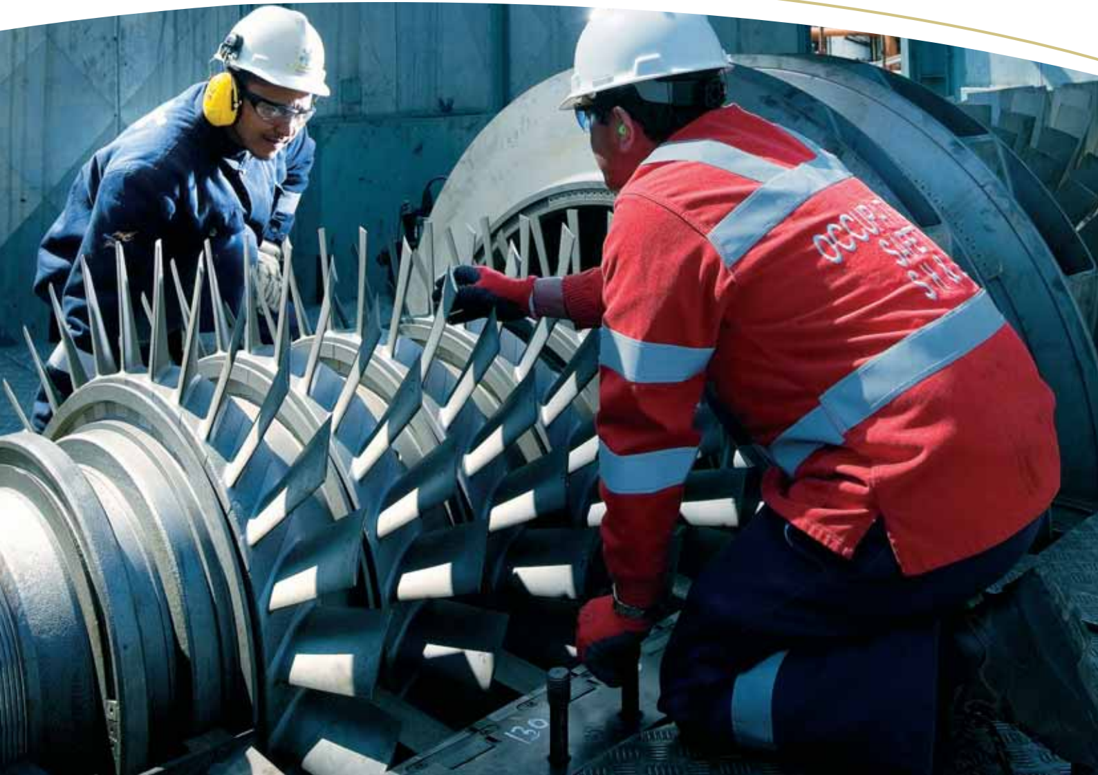
Turbine compressor at the oxygen west unit, Secunda.
