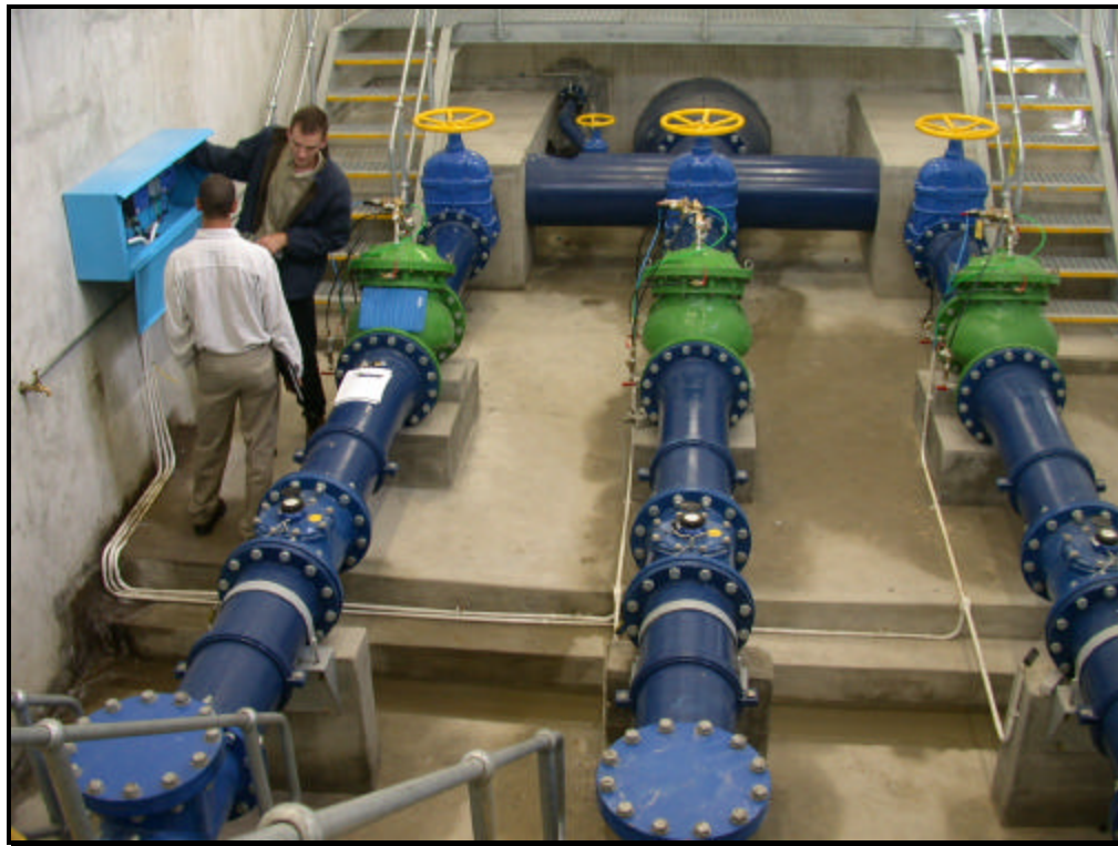
Figure 5: View Inside the Main Khyelitsha Pressure Management Chamber
