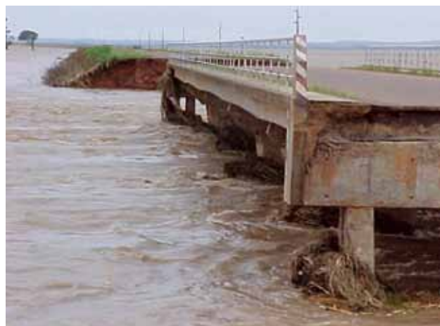
Figure 4.01: Flood damages to settlements and infrastructure
