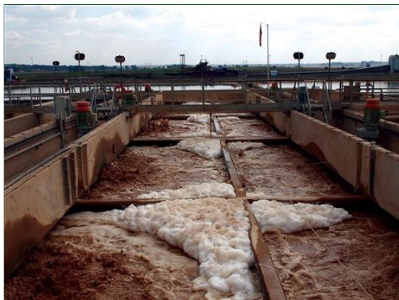
Oxide precipitation facility at Emalahleni, South Africa.
