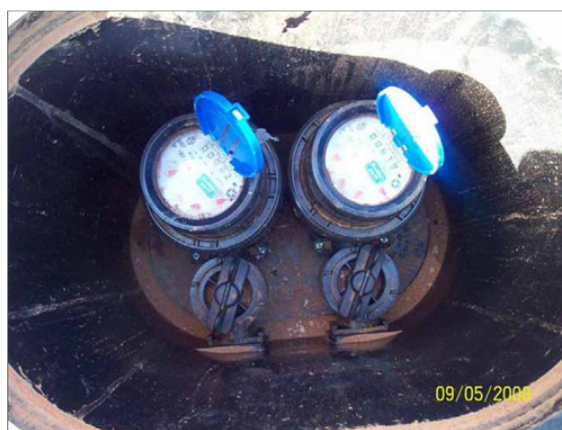
Water meters are one method of managing water control and utilisation.
