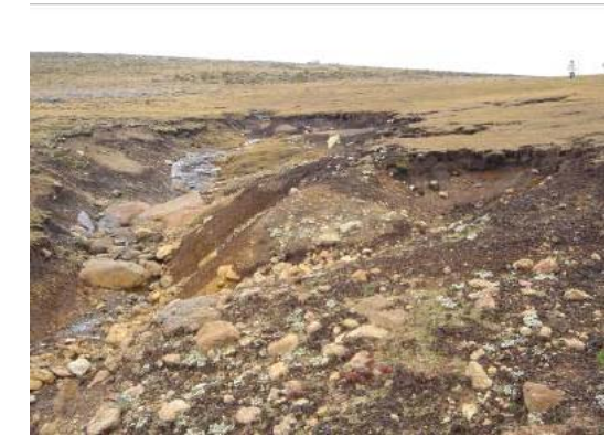
Erosion from road drainage
